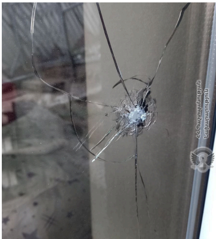
Damage to a residential building from the alleged 31 March shooting of Azerbaijani troop at the Khnatsakh settlement. Source: Ministry of Defense of Armenia
